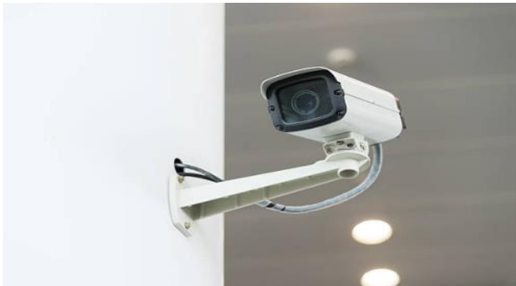
Risk: Unauthorized activities or theft Control: CCTV cameras
