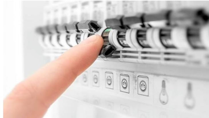
Risk: Short circuit leading to fire Control: Circuit breaker
